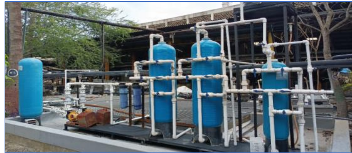
Acid Recycling used to recycle acid mixed water.
